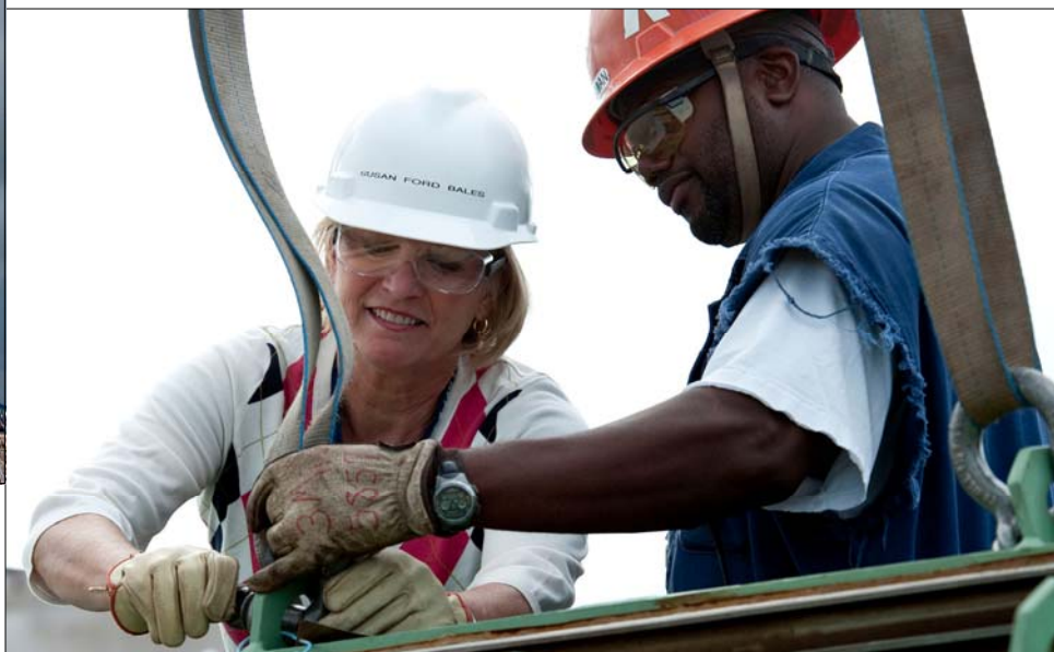
Susan Ford Bales, sponsor of the nuclear-powered aircraft carrier USS Gerald R. Ford (CVN 78) , assists shipbuilder Mike Jordan in a weapons elevator door installation.
